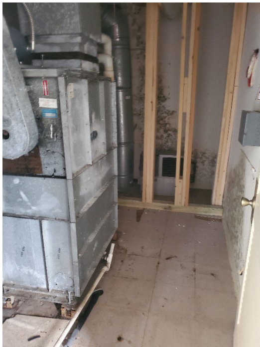
Figure 10. Cameron House Interior (HVAC Unit)
