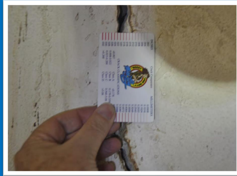
Cameron House (cracking)
