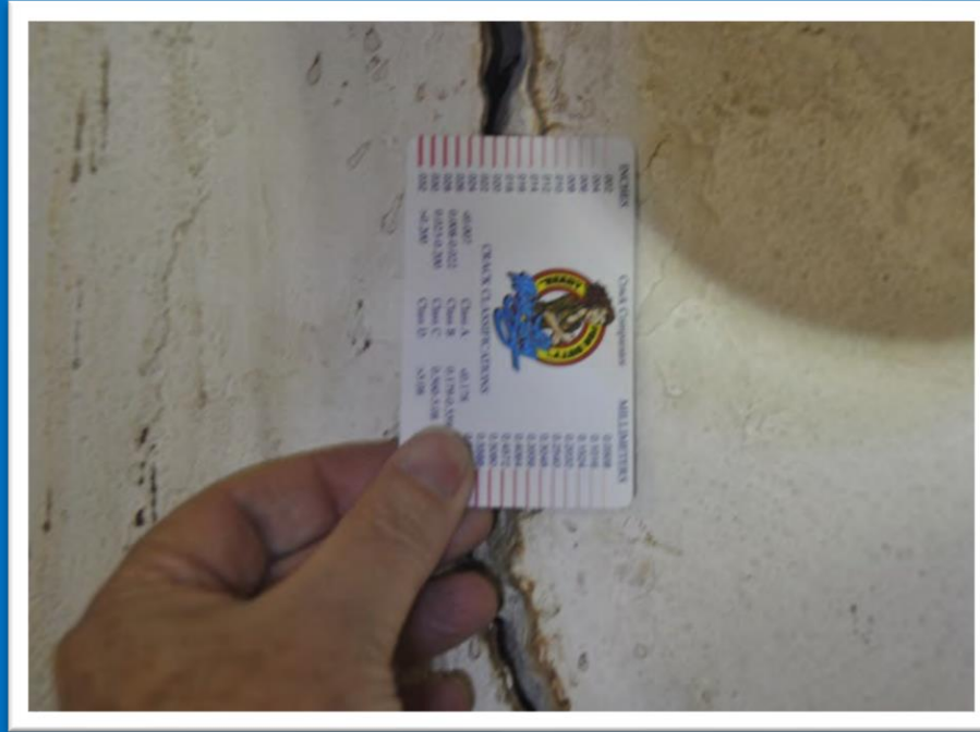
Cameron House (cracking)
